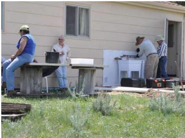
Putting in the new sink at Hell Gap, Stu and Barb Nahas and Don and Eva Peden.
